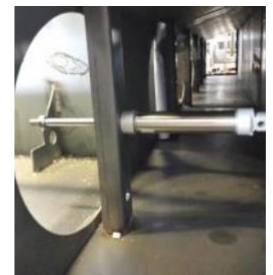
Valve evacuare fum
